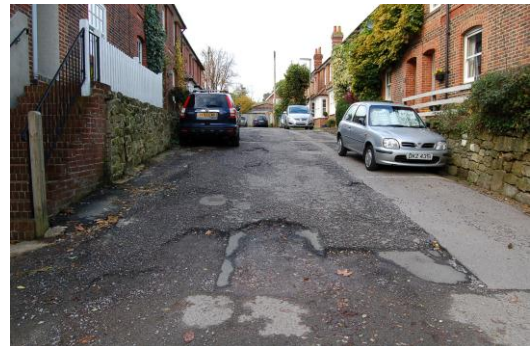
Figure 25: Road surface at Northfields
